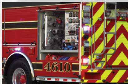
Operator's Side Pump Control Panel
