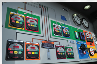
Logi-Color Pump Control Panel
