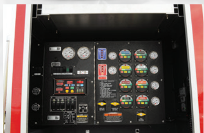
Curb Side Pump Control Panel
